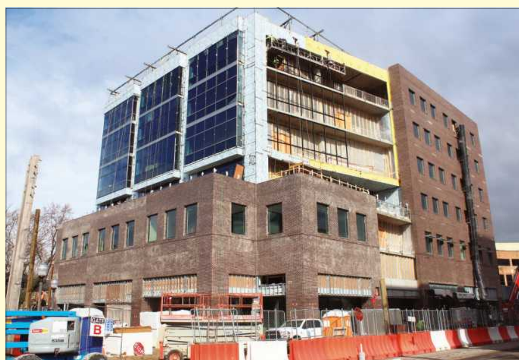
THE SEVEN-STORY building that will house Baker College in Royal Oak will have space for 1,500 students, adding significant vitality to the city’s downtown. Colasanti Construction Services is managing the project.
