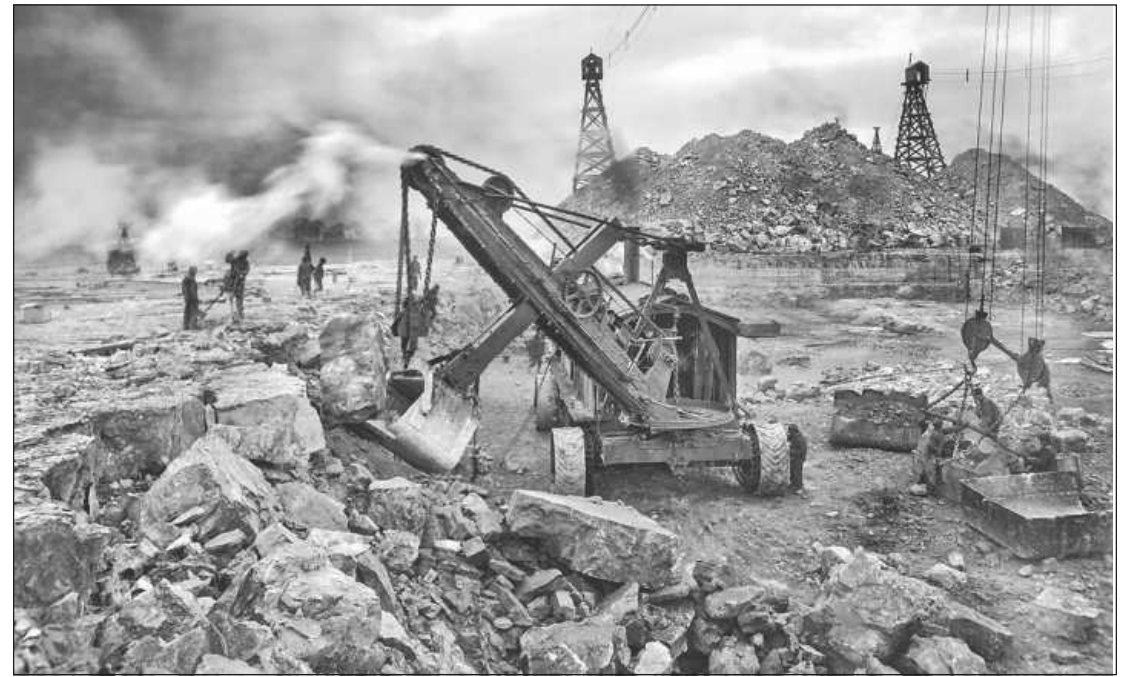
A STEAM SHOVEL removes rock loosened by dynamite in the Livingstone Channel, circa 1910. The Detroit River had been dewatered to allow for the massive project to deepen and widen the river.
