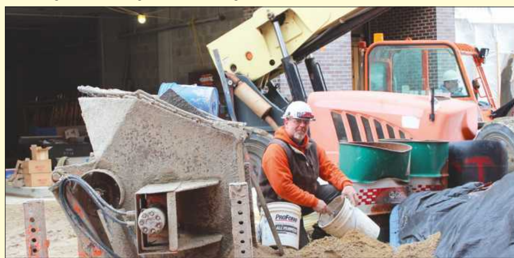
MIXING MORTAR for patch work at the Baker College project in Royal Oak is Scott Gillie of Bricklayers and Allied Craftworkers Local 2. He’s employed by Pomponio Construction.
